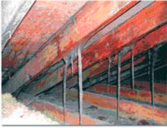
Condensation resulting from excess moisture being dumped into the attic has frozen on the underside of the roof sheathing
